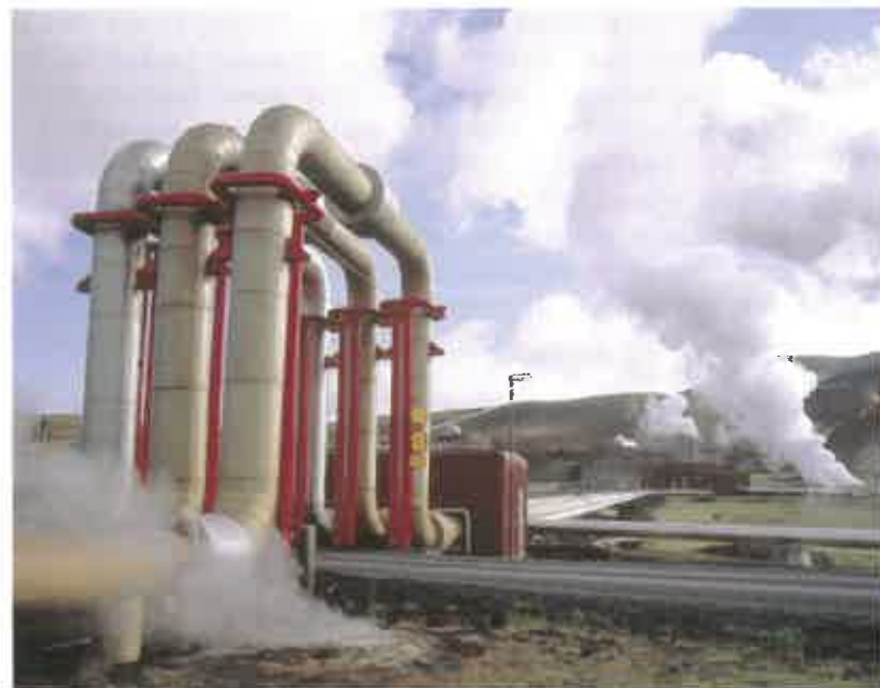
▼ FIGURE 9-47 GEOTHERMAL Geothermal plant near Krafla, Iceland.
